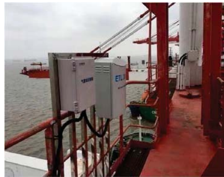
(Detecting device installed on shore crane)
